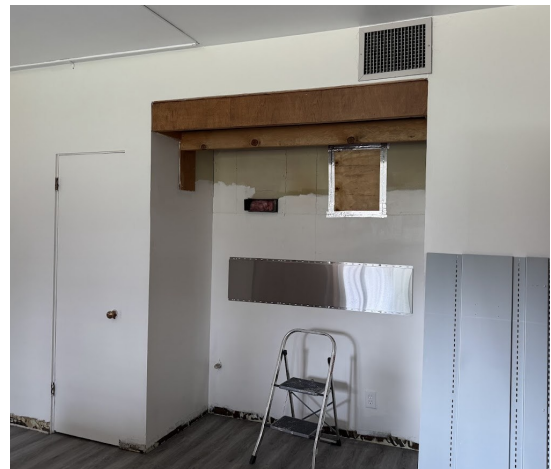
READY TO INSTALL THE NEW, GAS OPERATED, CHEF QUALITY STOVE!
